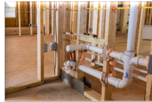
Figure 6: Water Distribution Pipes
